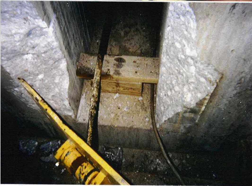
PHOTO: Damage to the gimbaled sheave pit and rope guide.
