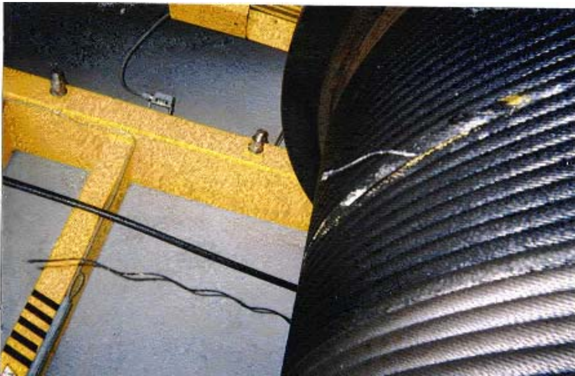
PHOTO: Damage to the steel wire rope.
