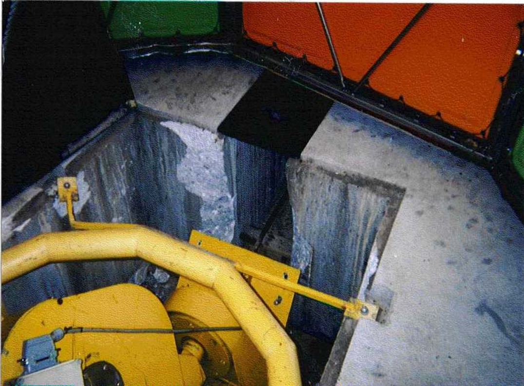
PHOTO: Damage to inner ring, support member and rope guide.
